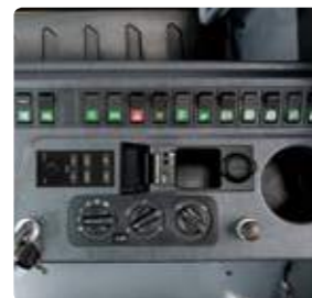
Centralized Instrument Switch Panel
